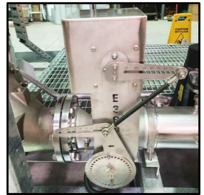
Modulating Control Valve
