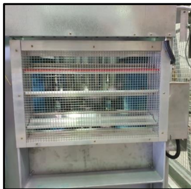
Automatic Air Dampers
